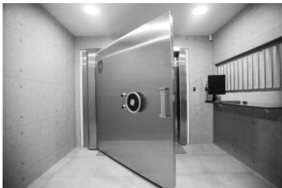
A 2.5 ton UL Class I Vault Door at TSH
